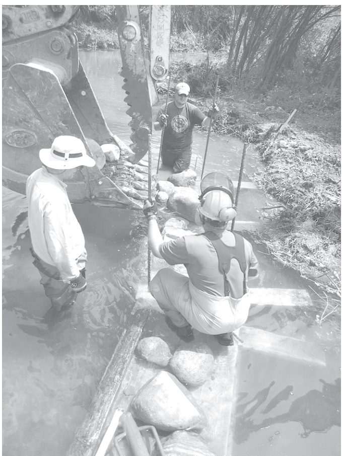
DEC Fishery Biologist Scott Cornett credits volunteers for the swift completion of the project. The fishing organization Trout Unlimited alone provided over 600 man-hours of volunteer labor.
